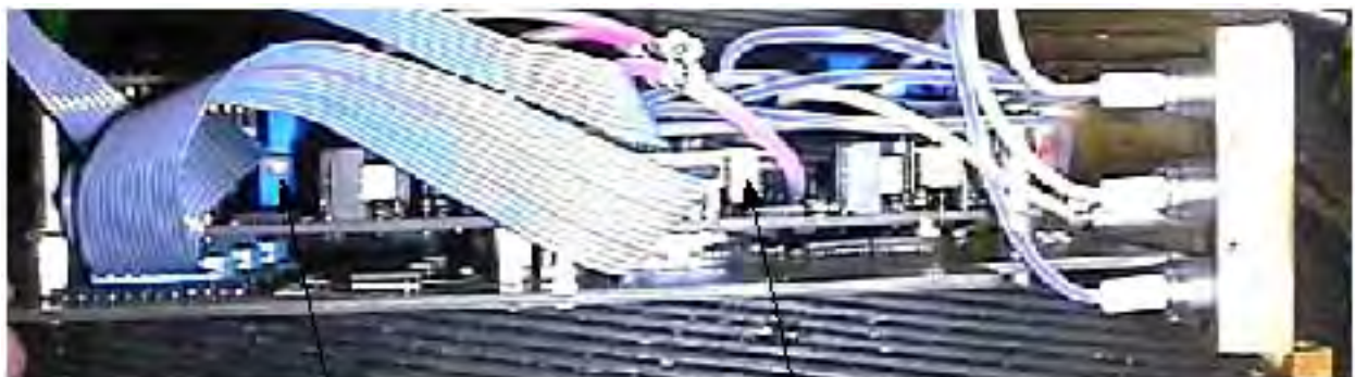
Figure 22 Maximum voltage adjustment potentiometers. The third is accessible from the other side.
